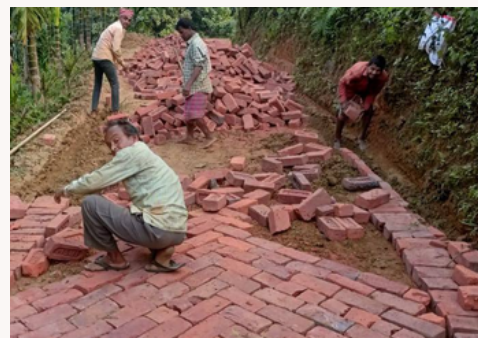
Brick Soling under FFC is being laid at Solonala VC, Pecharthal RD Block
